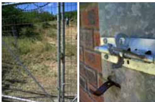
Figure 1.10.2: How access was gained and a lock hacked off the steel door at Mkhize Dam
