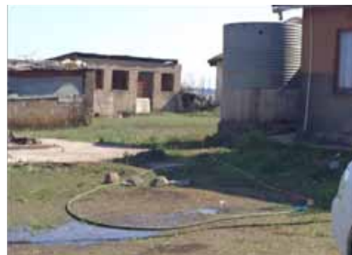
Figure 1.10.4: Water wastage at Mtimofu in uMlalazi Municipality, communal standpipe serving one household, illegally
