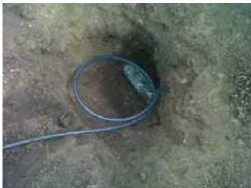
Figure 1.10.6: Ready for an illegal connection at one of our bulk lines
