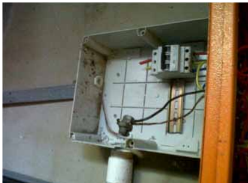
Figure 1.10.1: Vandalism of DB box at Mkhize Dam in Ntambanana
